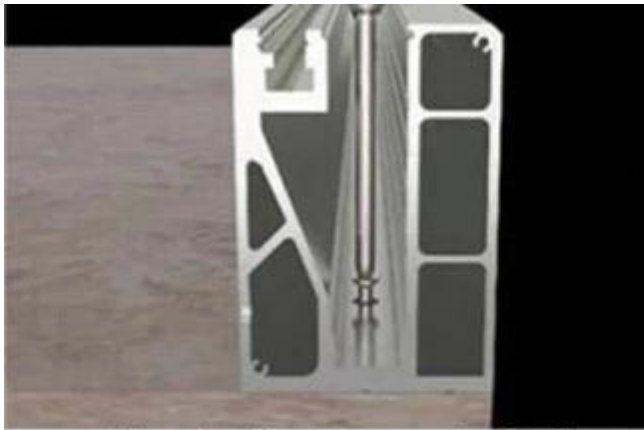
screw the aluminum groove to the floor and drill the drain hole
