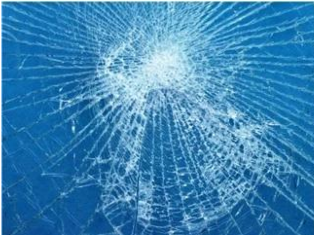
Non- tempered laminated glass broken
